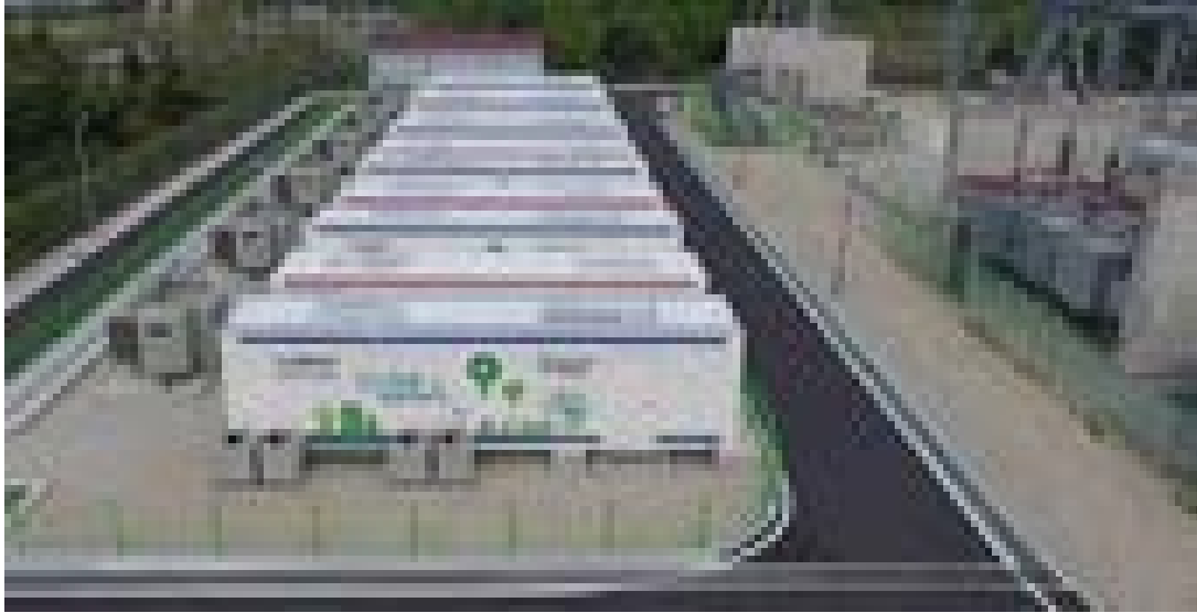
Figure D.4: Sokcho Battery Energy Storage System
